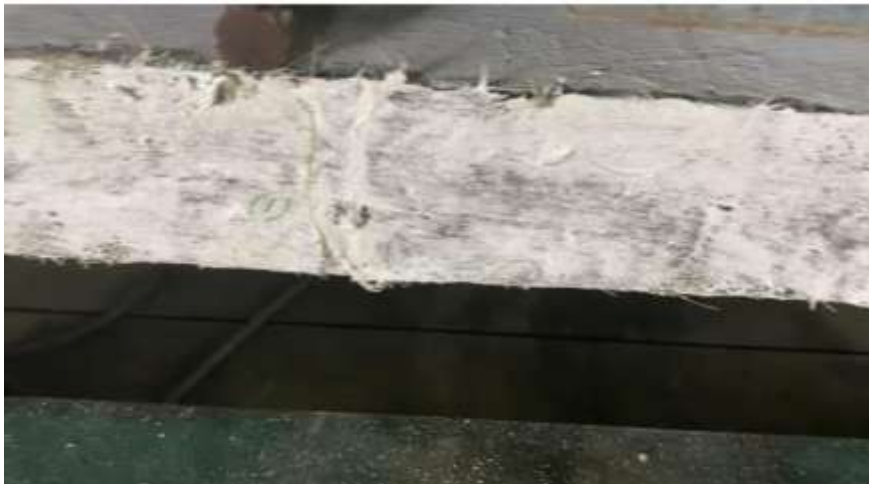
Fig ii4.4.4: iiCracked iipatterns ion iiU iiwrapped iicollapsed iibeam iiafter iiloading
