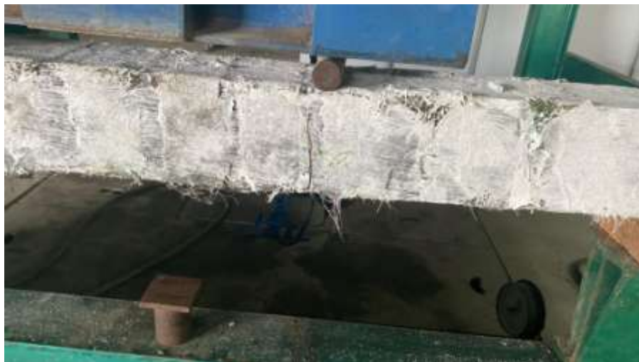
Fig ii4.3.3: iiCracked iibeams iiafter iiretrofitting
